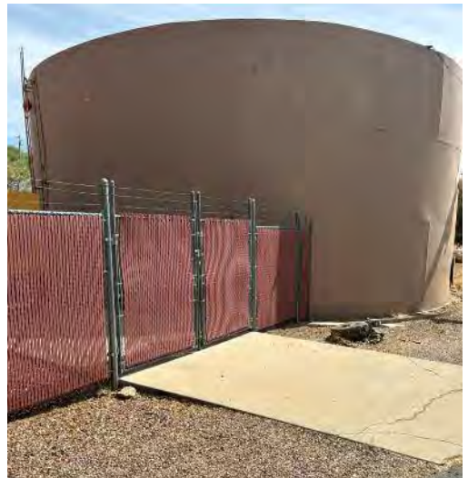
The 200,000 central distribution water tank
